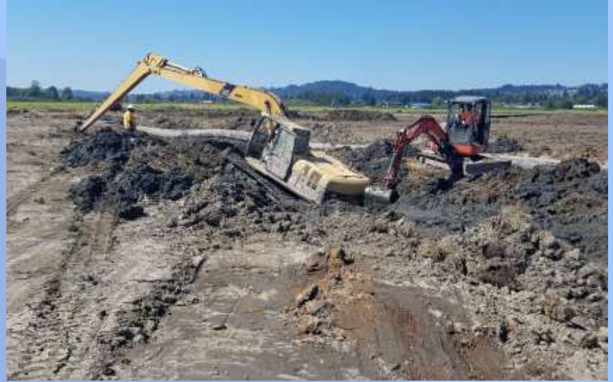
Heavy clay soils on site
